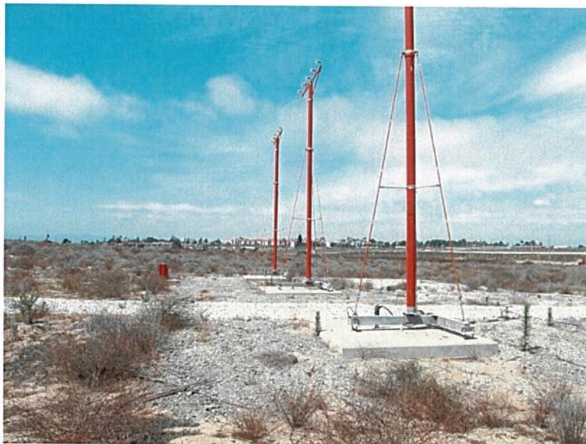
1000 foot light bar with steady burning lights to be relocated to the east of Pershing Drive. Concrete pads to remain in place.
