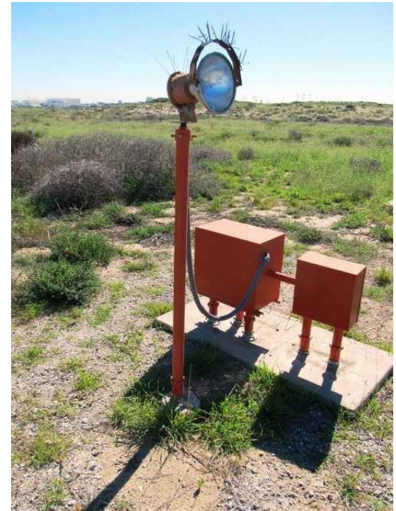
3. View of single-pole flashing station facing southeast.
