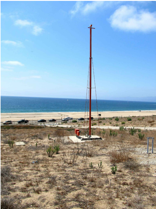
1. View of MALSR Station facing west.
