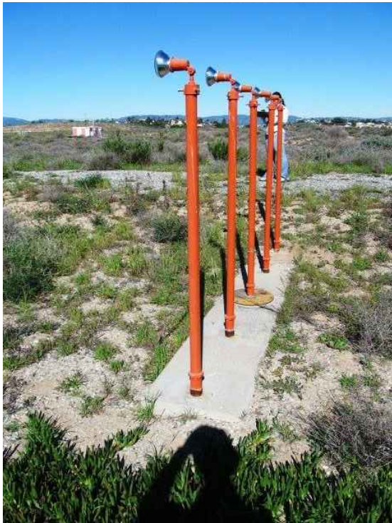
1. View of five-light steady burning station facing north.
