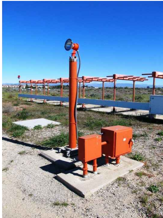
2. View of single-pole flashing station facing northeast. 1/
