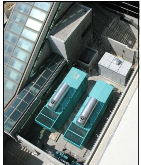
A pair of the new roof mounted air handling units.
