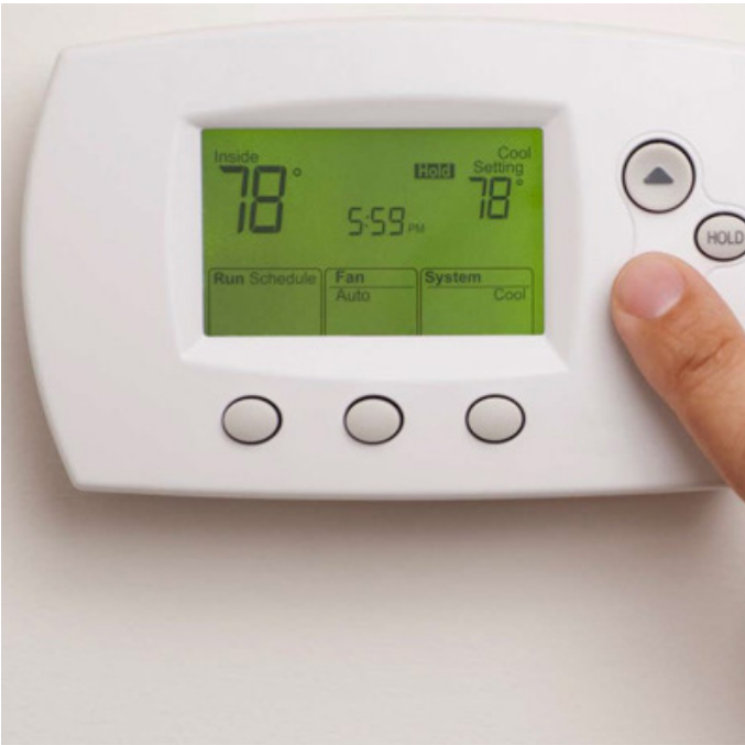
Thermal Control Source: www.climatecontrolme.com
