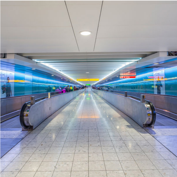
LED lights at Heathrow Airport Source: http://glamox.com/gsx/references/heathrow-airport
