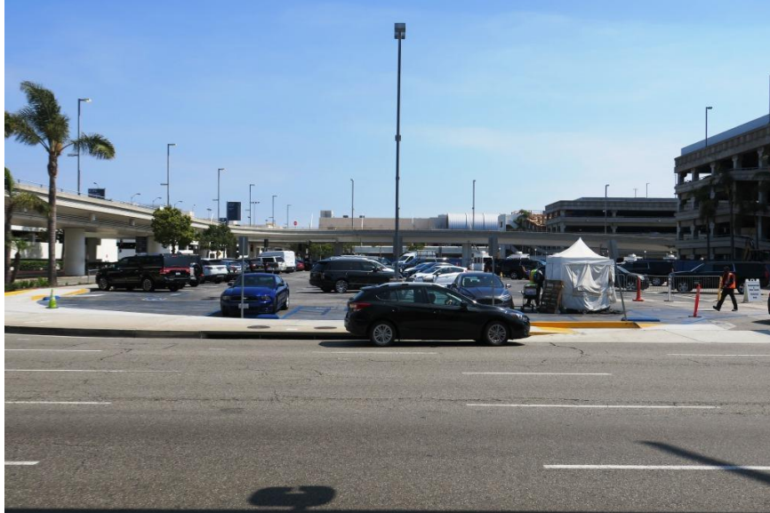
The surface lot next to Parking Structure 3 is closed for construction of a bridge from Terminal 3 to the Automated People Mover that will begin service in early 2023.
