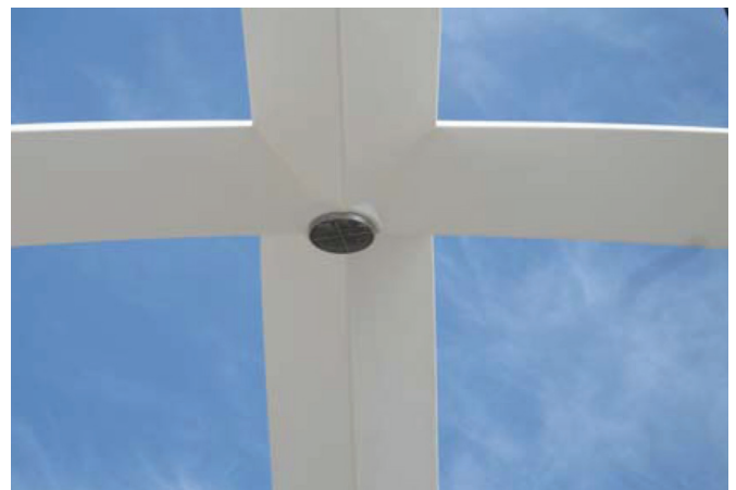
Air and moisture is expelled through this central vent to prevent damage from condensation.
