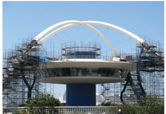
Arches of the LAX Theme Building undergo reconstruction with newly designed stucco to protect against rain and ice.
