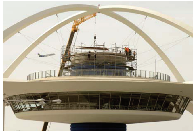
A Crane installs one of the 22 two-inch steel plates that comprise the tuned mass damper. A total of 600 tons of steel were placed into the top core as part of the unique seismic retrofit.
