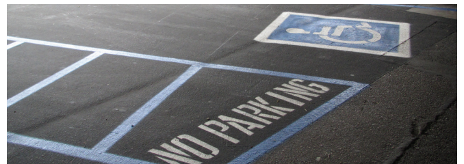
Repainting parking stalls is just one measure the two-phased ADA Improvements Project is undertaking to improve the passenger experience at LAX.
