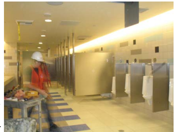
Restrooms at Terminal 1 have been upgraded with new fixtures, tiles and silvery metallic paneling
